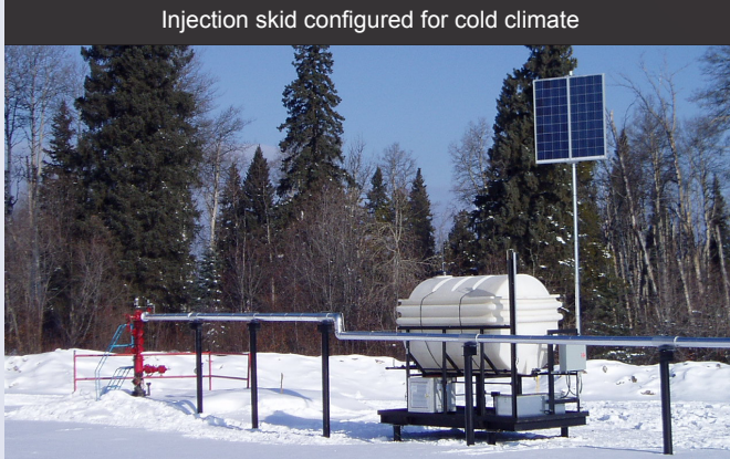
Injection skid configured for cold climate
