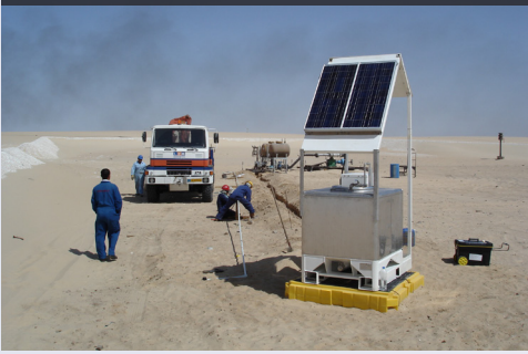
Injection skid configured for hot climate
